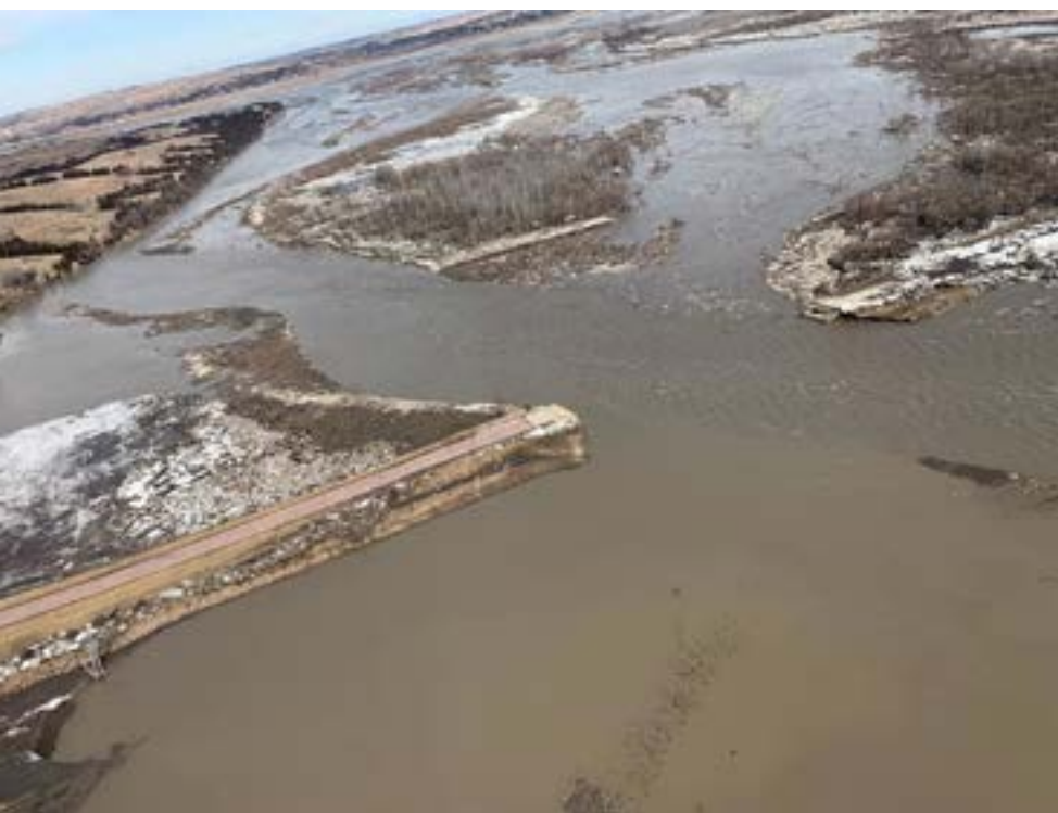
The Mormon Canal Bridge on Highway 12 near Niobrara, Nebraska, after the bomb cyclone hit on March 13, 2019. This bridge is near the confluence of the Niobrara River and the Missouri River. Niobrara State Park is on the left.
